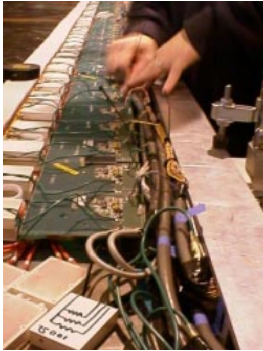
Figure 2: Amplifier/HV distribution cards installed in a panel.
